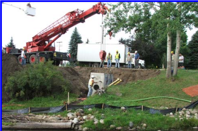
Above, an oil/grit separator, called a vortechnic unit, is being installed near the Au Sable River. This end-of-pipe treatment is used to complement the rain gardens and help filter out pollutants which would otherwise end up in the river.
